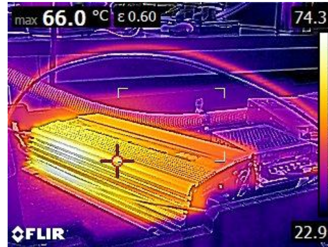
Fig 23: Thermal Image of the Inverter
