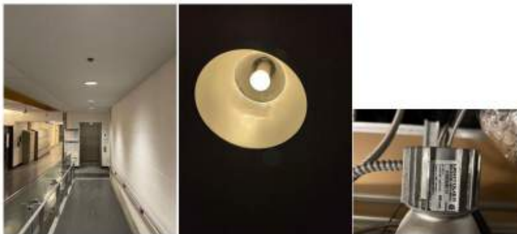
Figure 1-1 Existing Indoor Lighting: Lightolier - 71263242BG120 – 1 lamp 26W (C3)
