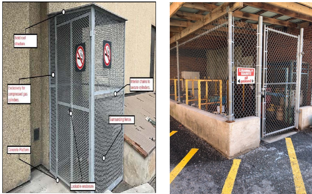
Figure 10 – Example of outdoor compressed gas cylinder storage requirements (rt photo storage by S&R)
